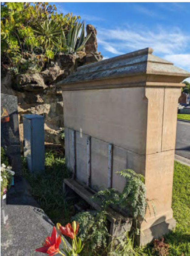
Figure 3 Rear view of trough showing remnant water pipes and vegetation
