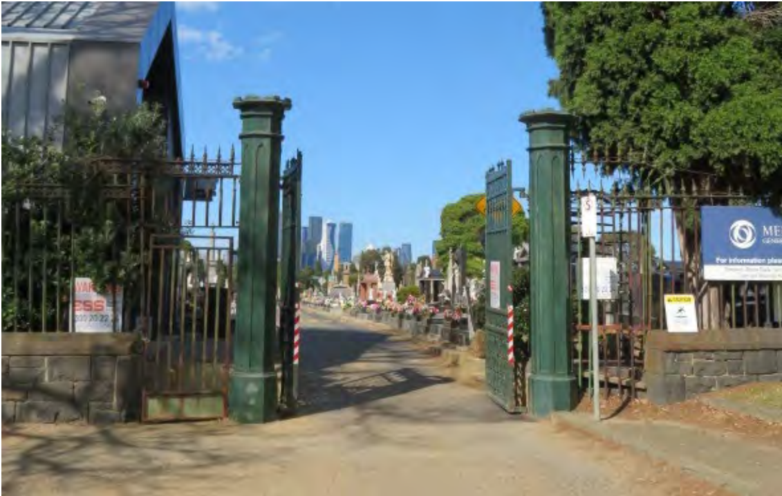
Figure 53 2023 condition of North Gate entrance, with inoperable pedestrian gates and a narrow shared entryway with no refuge or safety measures inside the cemetery
