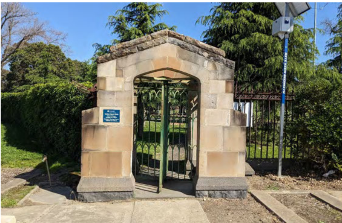
Figure 54 2023 condition of West Gate; in ground gravesites to both flanks limit options for creating a new barrier free access while retaining the original turnstile
