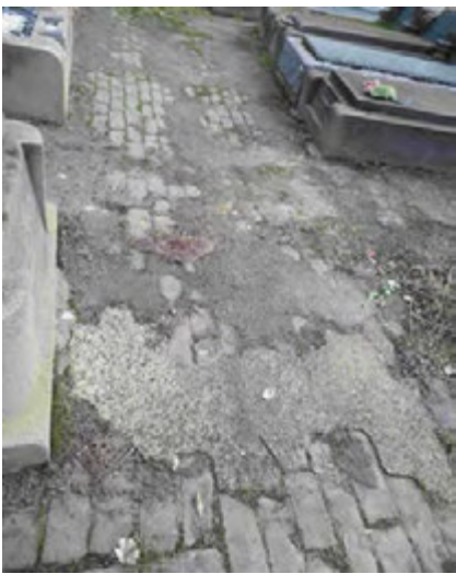
Figure 1 Remnant bluestone paver path with asphalt overlay
