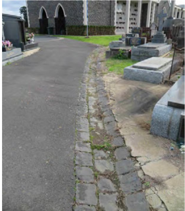
Figure 2 Bluestone three-pitcher drainage channel to the west side of Ninth Avenue looking towards the MGC Mausoleum
