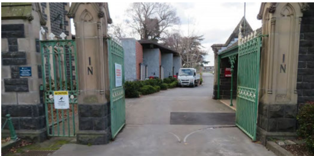
Figure 52 2023 condition of entry gate at main entrance, with pedestrian gate locked closed; a similar condition exists for the 'Out' gates
