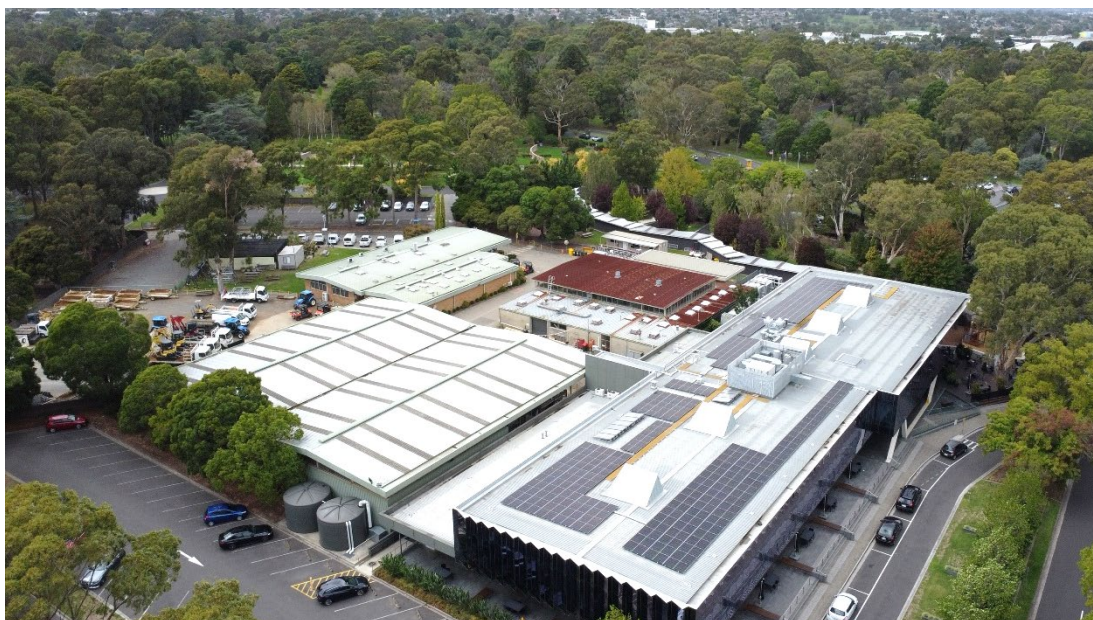
Solar power system at Springvale Botanical Cemetery
